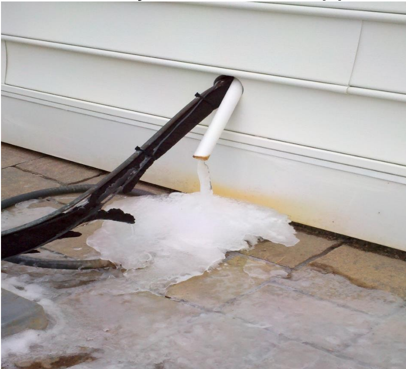
Photo #2 of badly frozen condensation pipe during winter of 2013-2014
