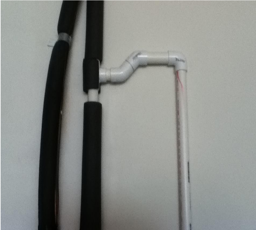
Photo #1 Converted Pipe
